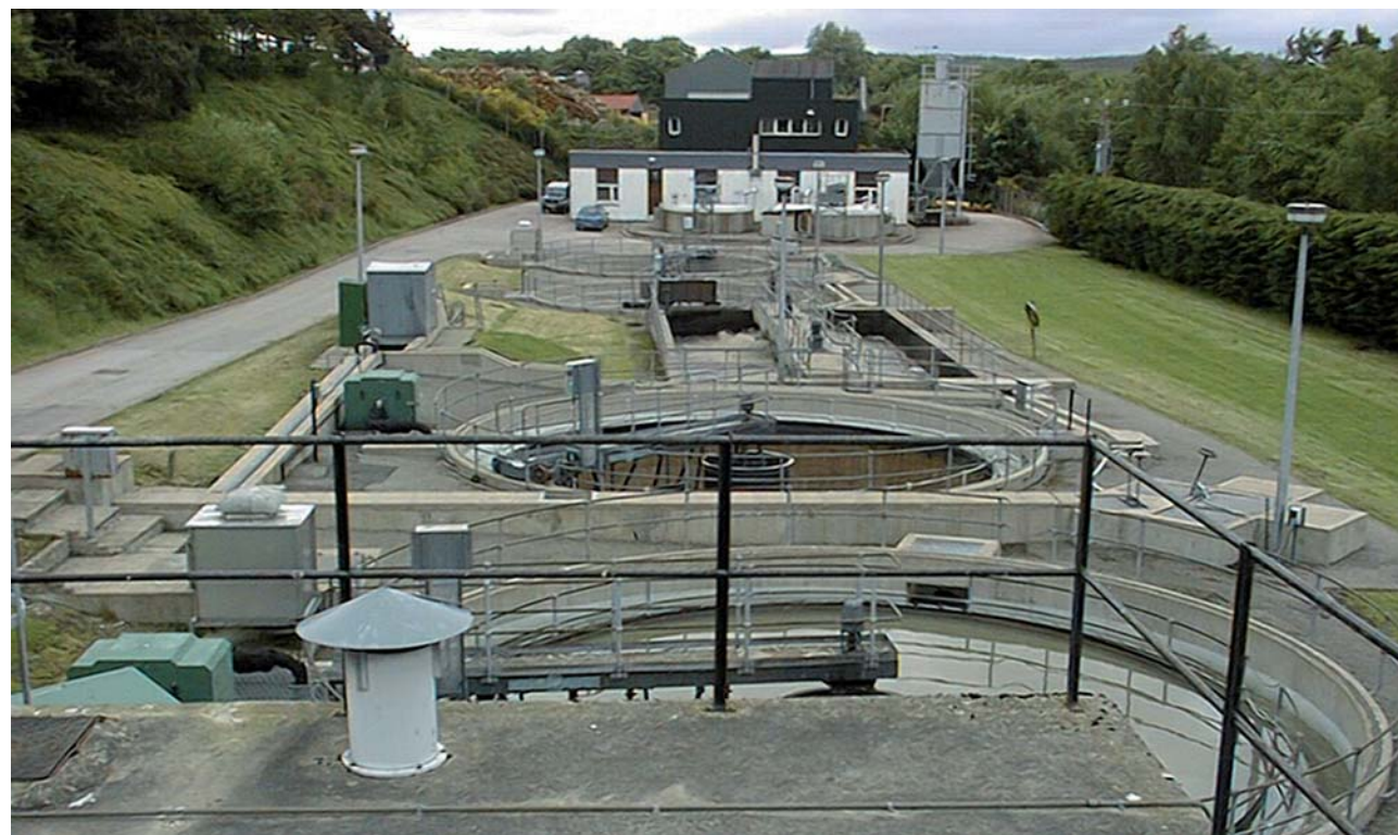
New Water Treatment Plant at Banchory (3 -Dee Vision)
