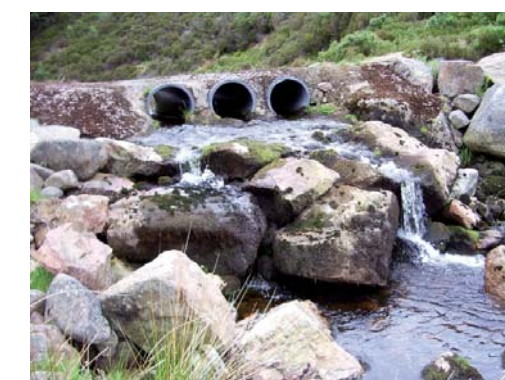
This pipe bridge on the Burn of Skinna (a tributary of the Water of Tanar) is impassable to fish (DDSF)
