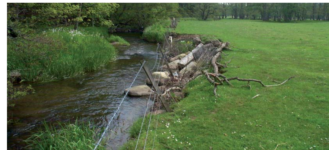
Unsuitable bank reinforcement works (Aberdeenshire Council)
